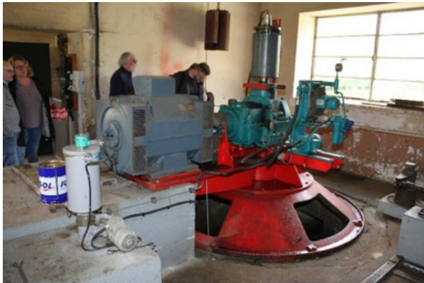
KAPLAN TURBINE INSTALLED IN 1946
