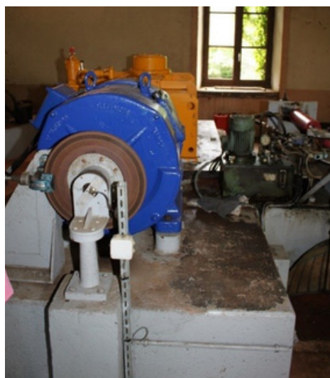
FRANCIS TURBINE INSTALLED IN 1961
