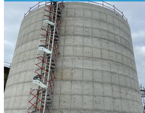
Sewage Treatment Plant
