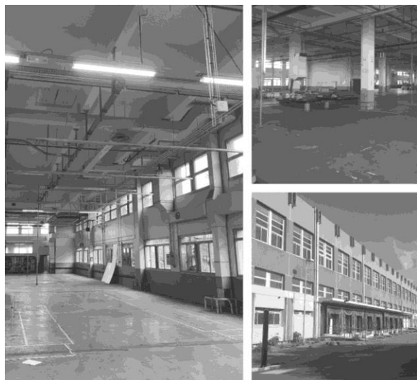
Current view of the former Amiens postal sorting center, the future PI 2 C
